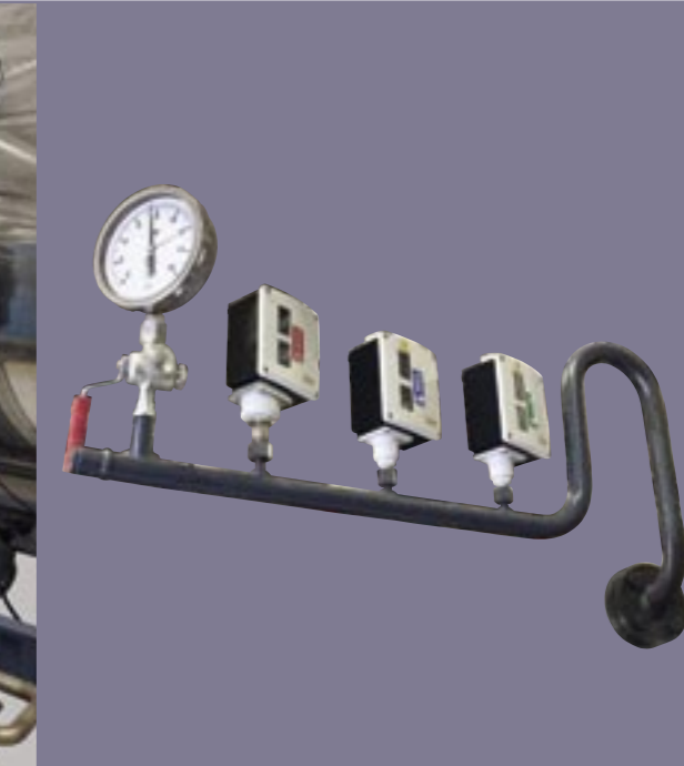
pressure gauge and switches cock
